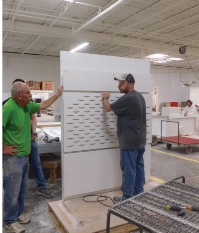
Deliver components to site and segregate. Note identification markings on each component.
