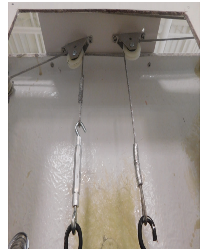
Note Location of cables inside of hood.
