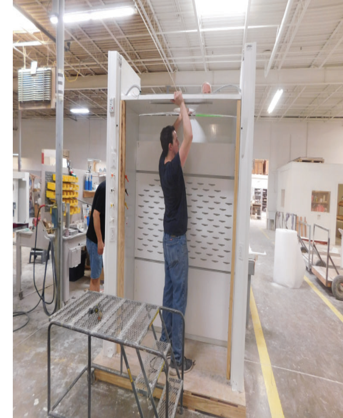
Front should be supported by bracing or personnel until Ceiling Panel is secured along the left and right sides to both the Side Shells.
